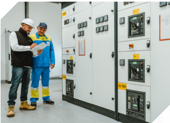
Schneider Electric solutions helped Danone Evian upgrade its bottling facility.
